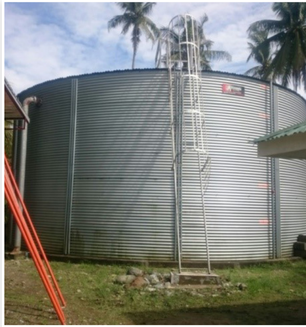
Km 6, Libertad Ground Reservoir and Booster Station
