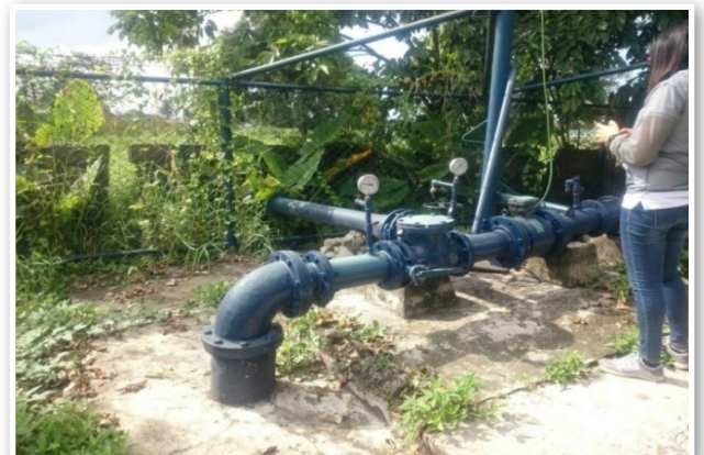
Pump Station No.03
