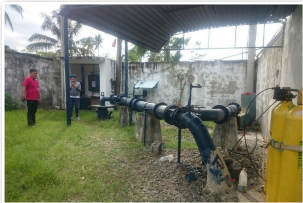
Pump Station No.15
