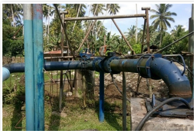
Pump Station No.15
