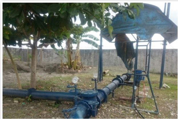
Pump Station No.14
