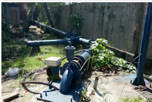
Pump Station No.01
